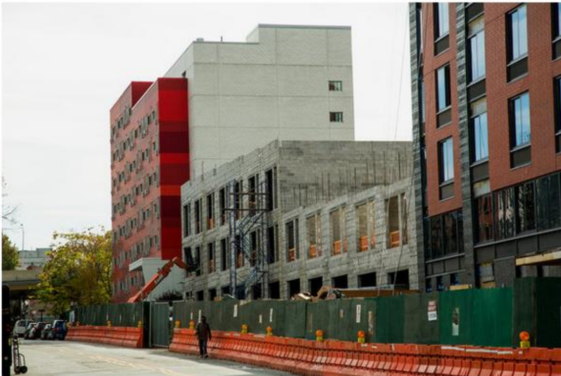
Construction at the Navy Green housing complex. Pablo Enriquez for The New York Times
